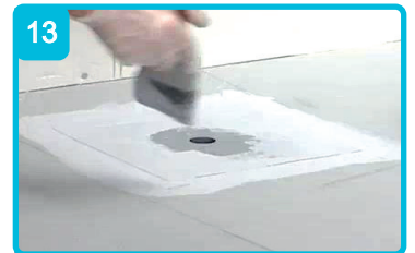
Brush out any creases and excess compound. Apply a coat of compound over the complete area. Leave to dry.
